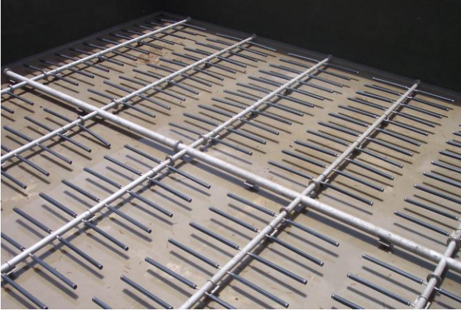
Fig. 4 Empty Aeration tank (Air diffuser pipes)
